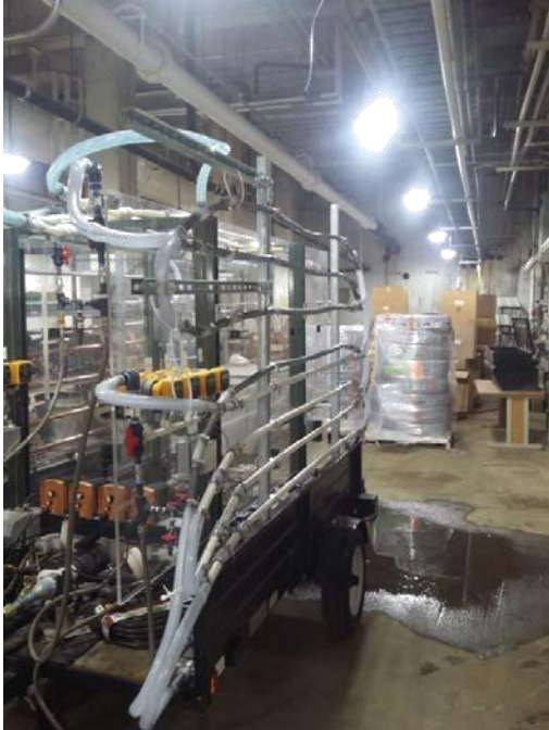
Figure 2: Pipe loop displaying PEX-A train (on top of pipe loop), Galvanized Steel train (top of loop wall) and Copper-K train (bottom of loop wall).
