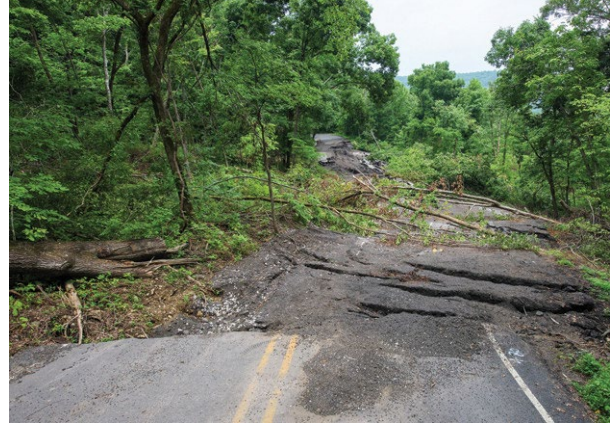
(B) Landslide on Highway 23 in Arkansas, August 2015 (Ref: Arkansas Business)
